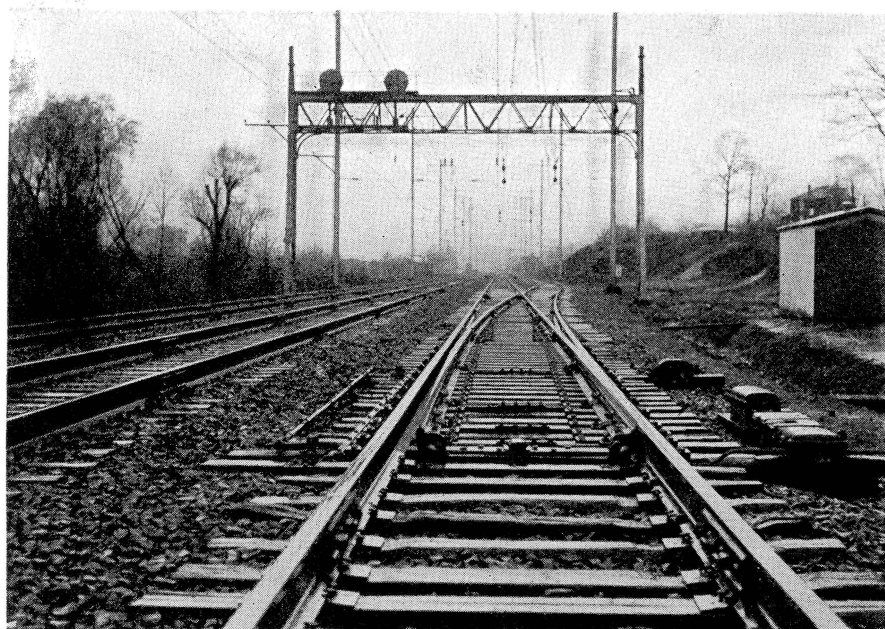
Signals and power switches at Winans with concrete instrument house in background
