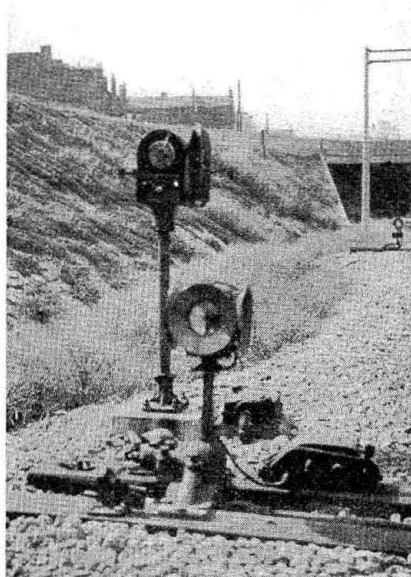
Switch indicator and time-element release at switch
