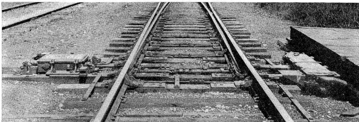
The junction switch at Duck Creek is power operated by means of a Model-5A machine equipped with dual-control selector
