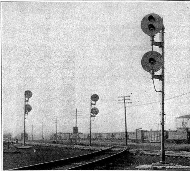
G-R-S two-indication color-light home signals are located about 35 ft. from crossing
