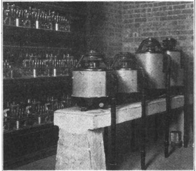
Above, Fig. 10—Motor Generators and Switchboard Below, Fig. 11—Portion of Relay Cabinet to Left
