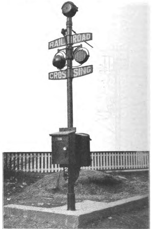
Installation of Nachod Flasher Light Crossing Signal on P. R. T. Lines
