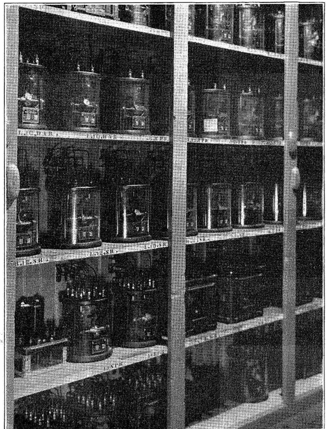
A Portion of the Relay Case in the Newark Plant
