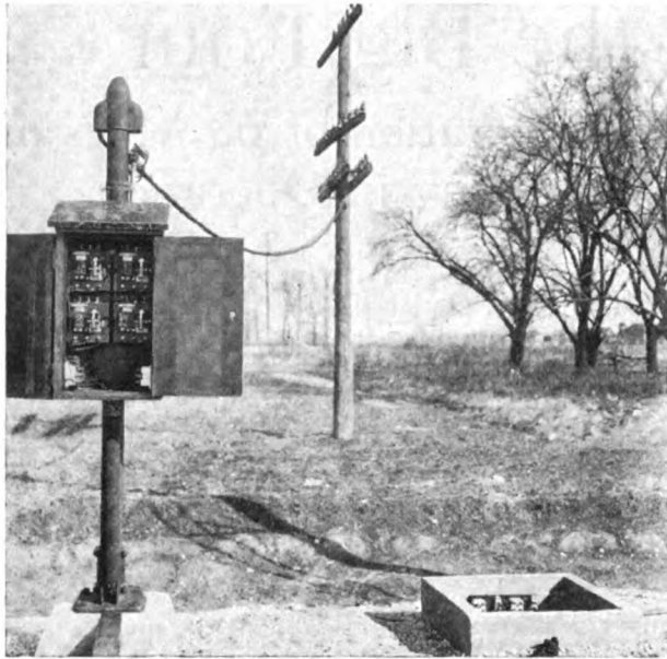
All Rectifiers at a Signal Location Are in One Box
