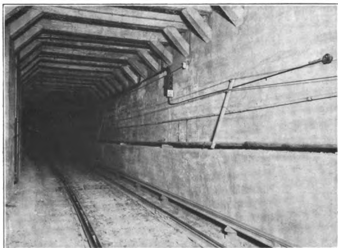
Fig. 12. Automatic Signal Location and Automatic Stop Release Box.
