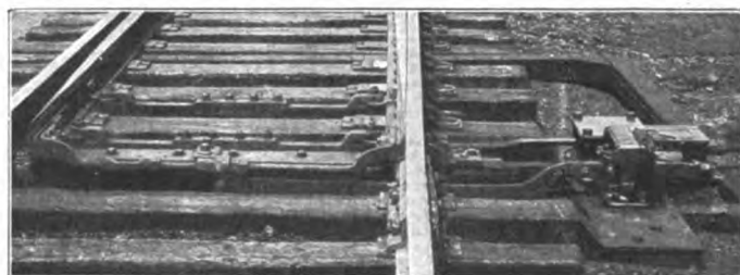
Fig. 6. One of the Switch-and-Lock Movements Installed at Trenton.
