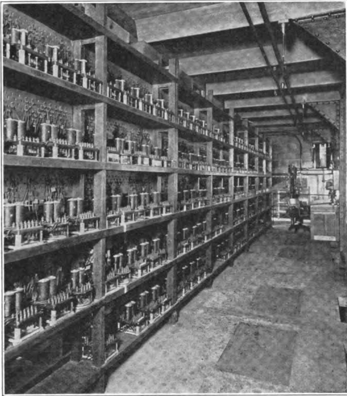
Relay Rack on First Floor of Tower A.
