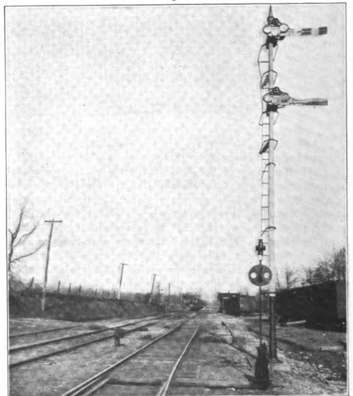
Double-Blade Home Signal Governing Crossover and Wye Switch.
