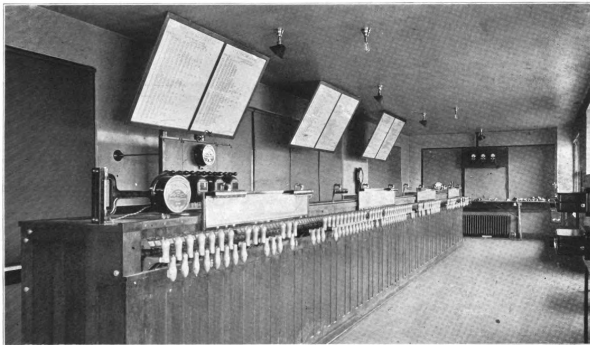
Fig. 1. Operating Room on Second Floor of Tower, Showing Lever Lights and Illuminated Track Diagram.
