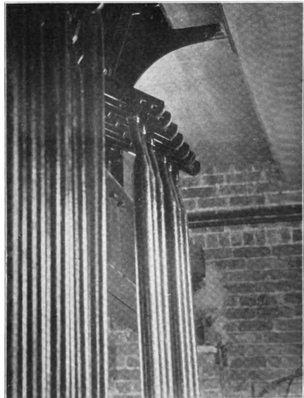
Fig. 10. Showing the "I" Beam Machine Support in the Clinton Junction Tower, and the Heavy Up-and-Down Rods.
