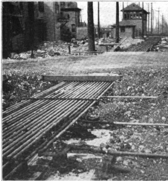
Fig. 5. Pipe and Wire Lines Under Street Crossing.
