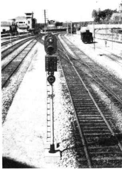
Fig. 4 X 3801 Main signal with luminous sign
