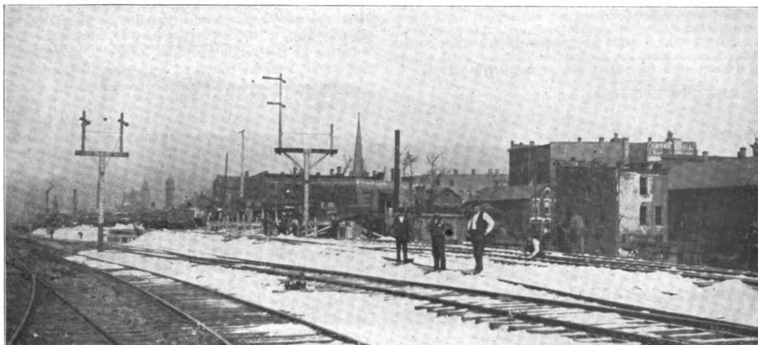
TRACK ELEVATION IN CHICAGO—BEGINNING OF WORK ON THE SANTA FE, ALTON AND ILLINOIS CENTRAL BETWEEN CHICAGO RIVER AND STARK STREET.
