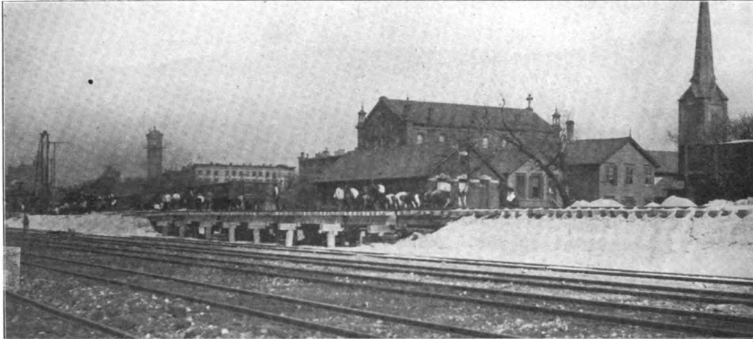
TRACK ELEVATION IN CHICAGO—BEGINNING OF WORK ON THE SANTA FE, ALTON AND ILLINOIS CENTRAL BETWEEN CHICAGO RIVER AND STARK STREET.
