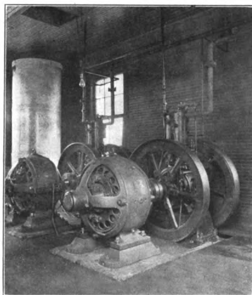
Power House for Signals at Sixteenth and Clark Streets, Chicago.
