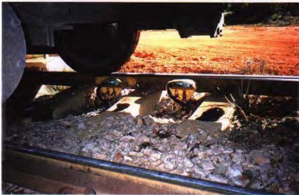
Figure 16: Proximity switches on loop.
