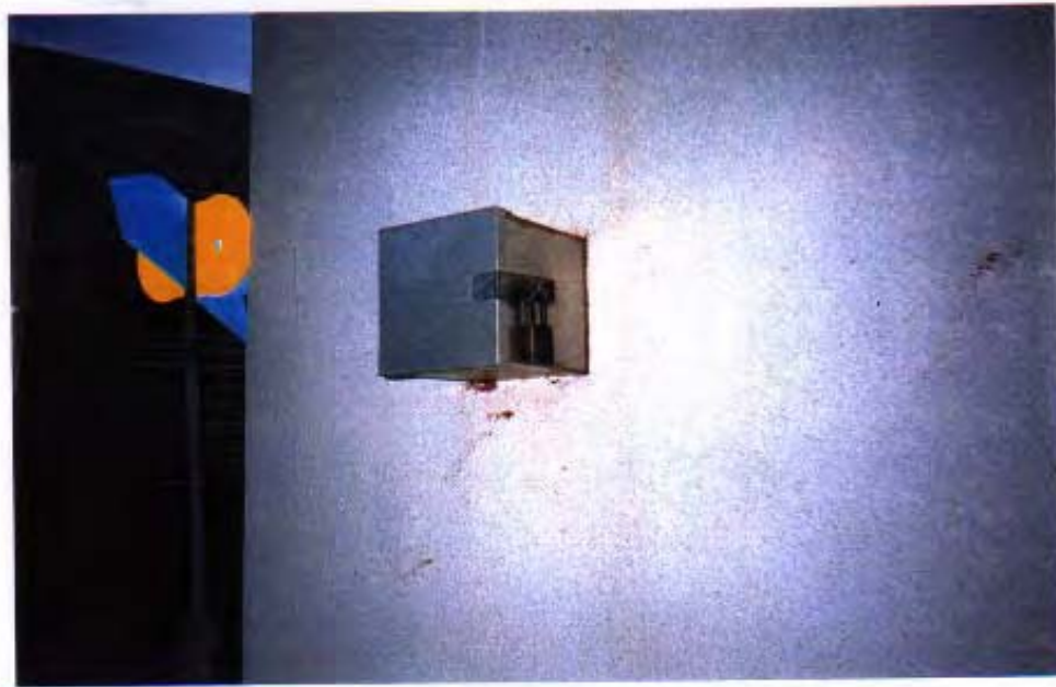
Figure 6: View of locked push button control box and yellow dumb bell indicating points set for loop
