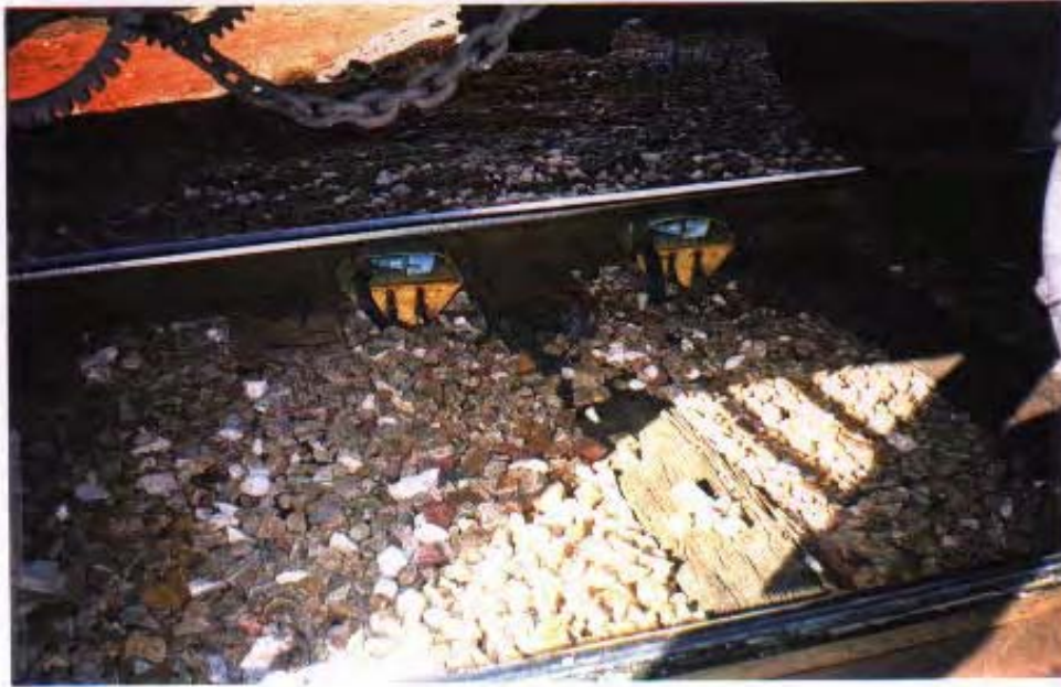
Figure 15: Proximity switches on main.
